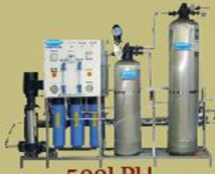
500LPH RO Plant
